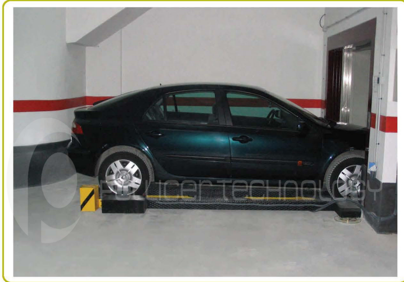
SITUATION : EXIT-ENTRY TO CAR LIFTING PLATFORM
